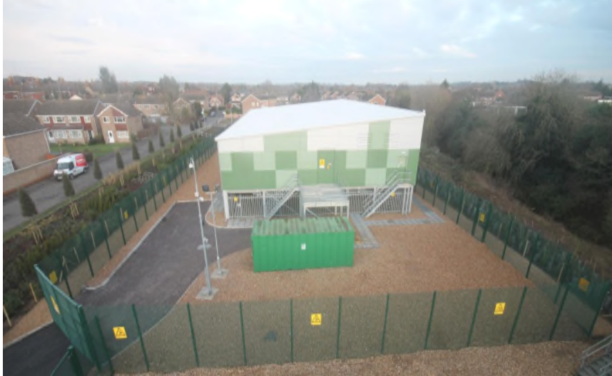
Image 1 (courtesy of UKPN): Smarter Network Storage (SNS) at Leighton Buzzard (6MW, 10MWh, Li-NMC).
