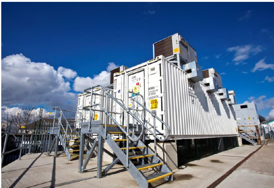
Image 3 (courtesy of NPG): Battery storage unit at Rise Carr, Darlington
