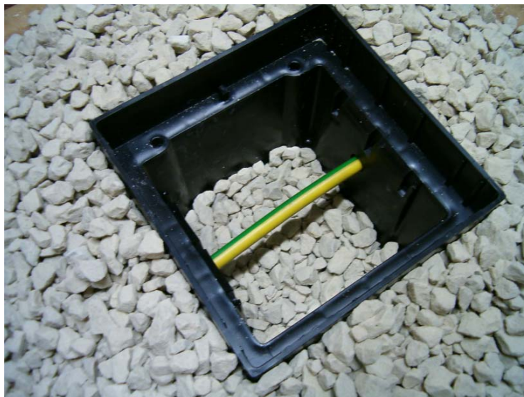
Figure 1 An example of earthing connection box with test facility*
